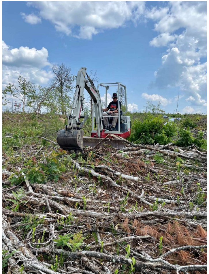
Trail Boss Jack Potter clearing tree tops from the area for the new trail on the McKenna Loop. Photo by Cortney Higgins.
